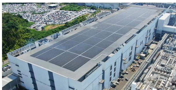
Solar power generation system at Kioxia Corporation's Yokkaichi Plant (Fab 5)
