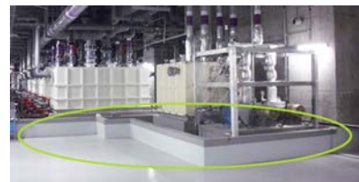
Drainage dike Prevents wastewater from leaking underground or into public water areas.
