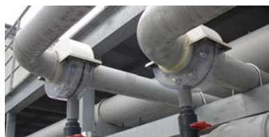
Double piping joints Monitoring and prevention of liquid leakages
