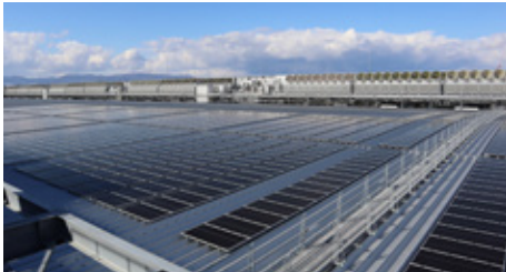
Solar power generation system at Fab1, Kitakami Plant
