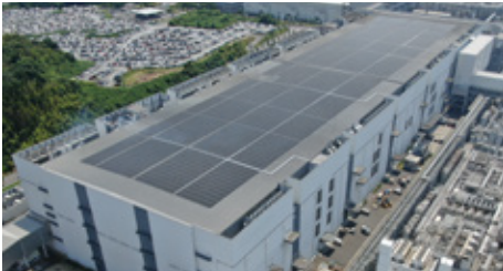
Solar power generation system at Fab5, Yokkaichi Plant
